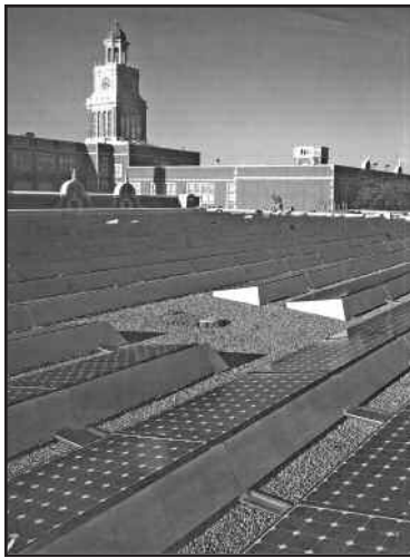
Solar panels have been added to the rooftop of the Panek Gymnasium at East.
